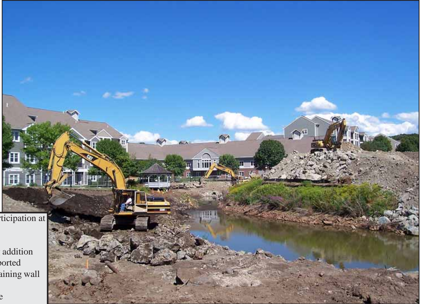
C.E. Floyd Company is adding 48 independent living units with an underground parking garage;
